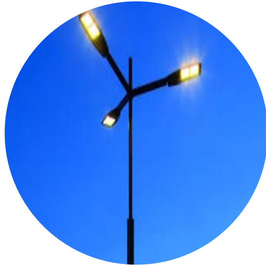
Eclairage public: 2 GWh
